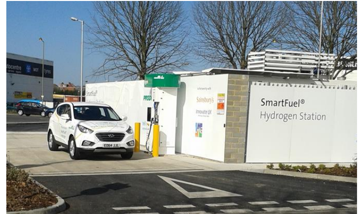
Hydrogen filling stations
